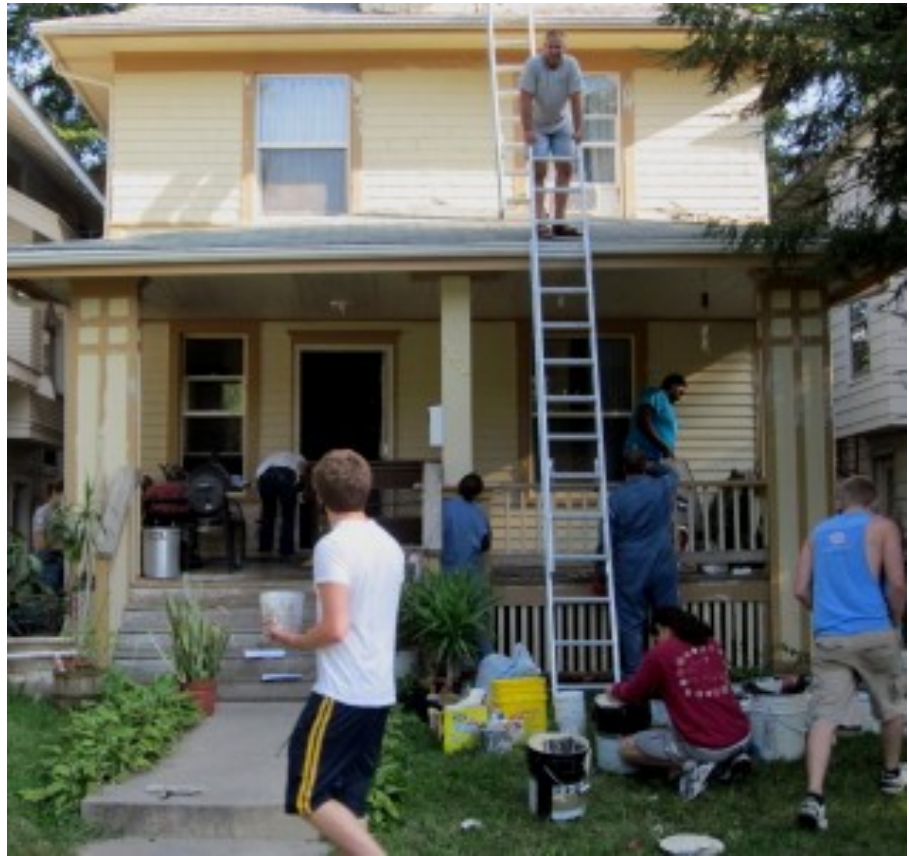
NCCC volunteers and BRIGHTEN staff help to restore a house in Wellington Heights.
